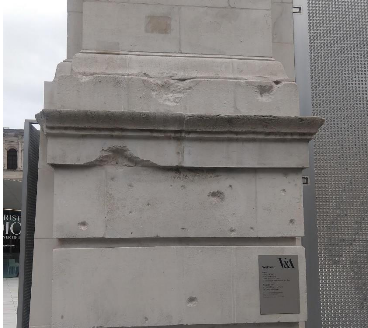
Figure 25, Photo of war damage to Aston Webb Screen alongside perforated metal gates.
