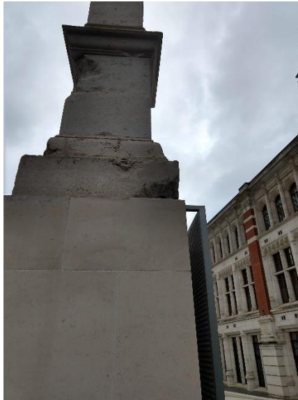
Figure 29, Photo depicting both original (top) and replacement (bottom) stone on Aston Webb Screen. Original in colour.
