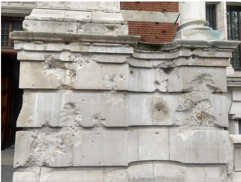
Figure 2, Photo of blitz damage to Exhibition Road facade of V&A. Bomb impact marks can be seen as varying in size and shape.
