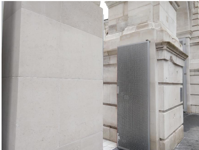
Figure 30, Photo depicting original (right pillar) and replacement (left pillar) stone on Aston Webb Screen. Original in colour.
